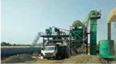
Hot / Batch Mix Plant
